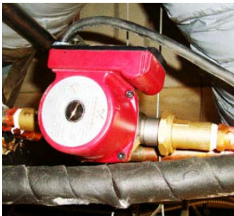
Figure 250 가압 Booster Pump
