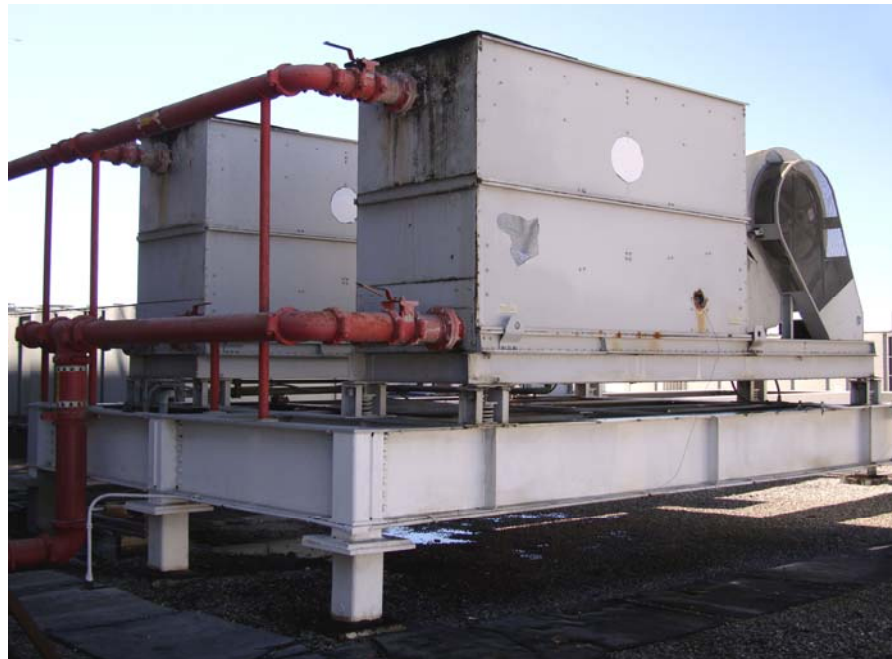
Figure-16-3 Water Cooling Tower
